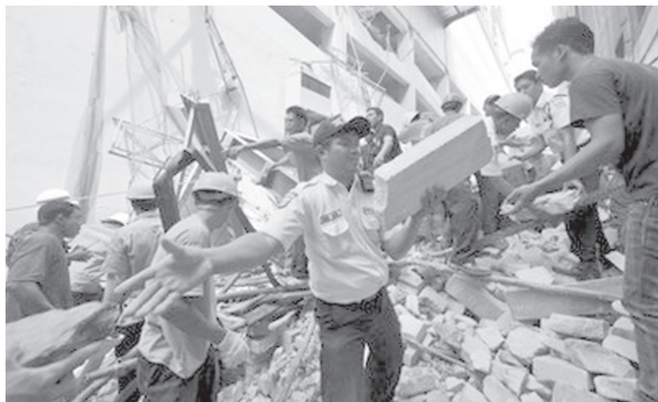
Three people were killed and 13 were injured after a building collapsed in central Jakarta on 23 December, according to police. City officials said the building, which was still under construction, was an unauthorized annex to a shopping mall.—INTERNET
