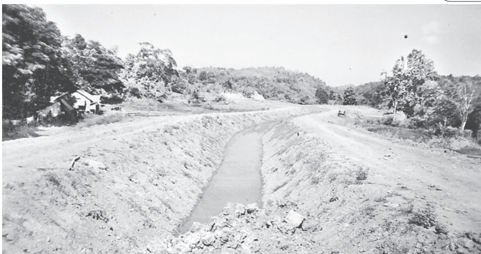
The left tributary under construction is meant to irrigate some 1000 acres of summer paddy.
