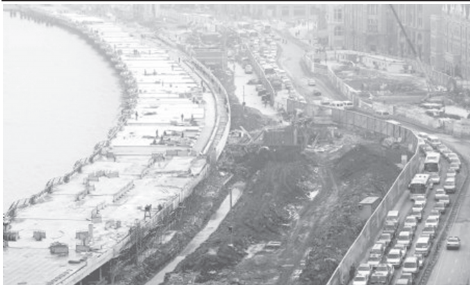
The photo taken on 17 Dec, 2009 shows the sight-seeing platform and driveways under reconstruction in the Bund by the Huangpu River in east China's Shanghai Municipality. —XINHUA
