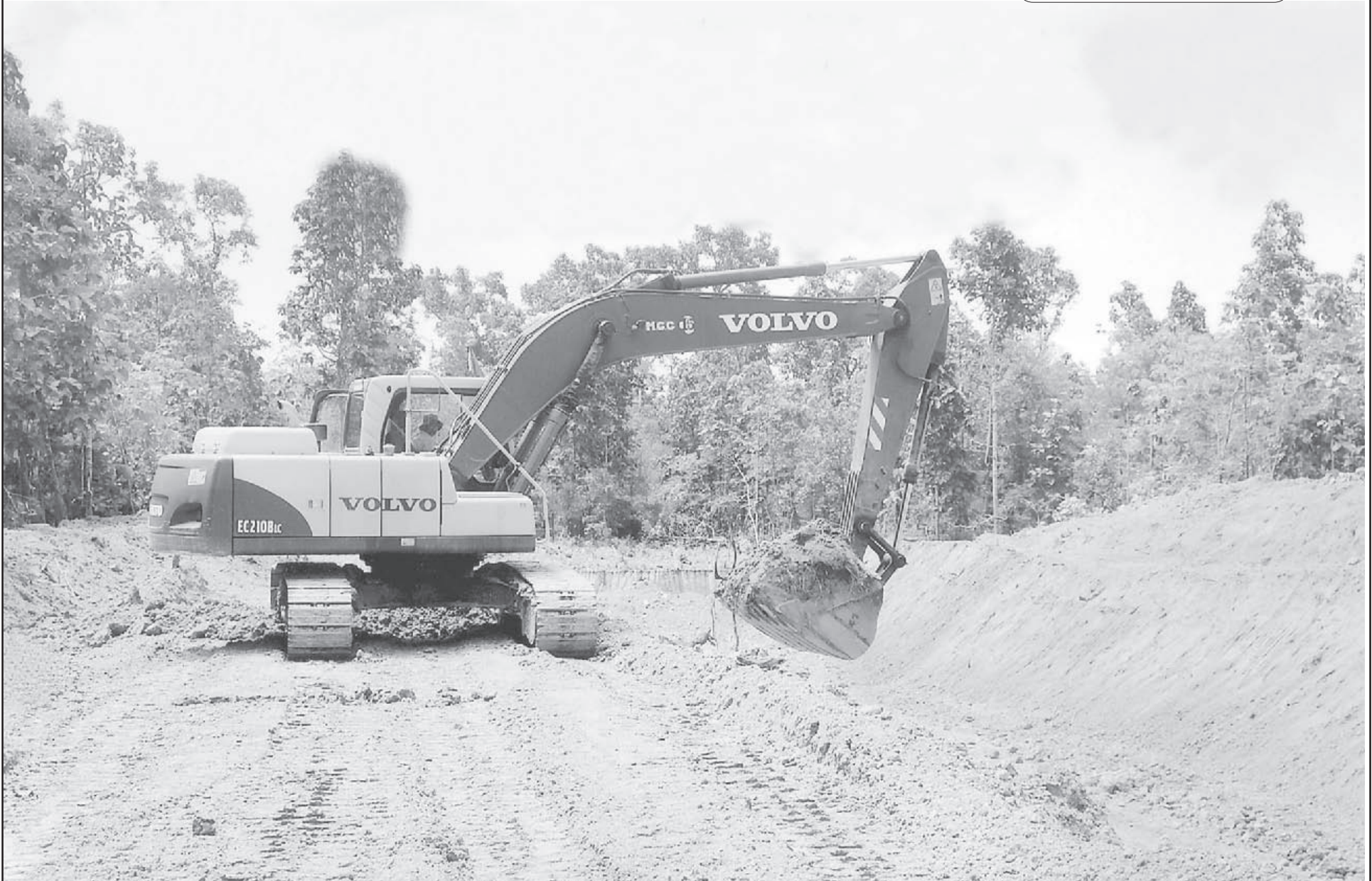
Construction of Katha-Bhamo railroad section in Shwegu Township of Kachin State in progress.
