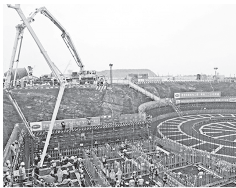
The photo taken on 15 Dec, 2009 shows the construction site of the second of the two generating units of the Sanmen nuclear power plant in east China's Zhejiang Province. XINHUA
