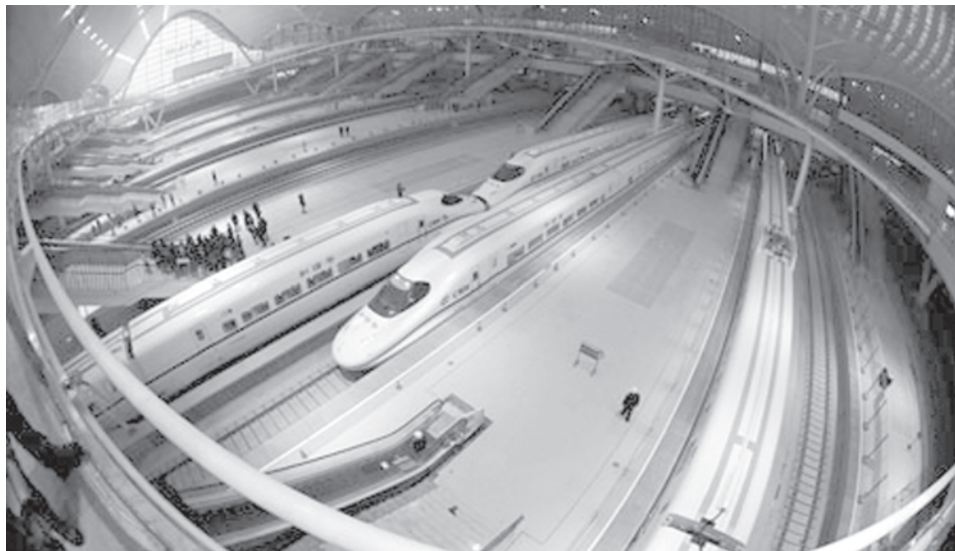
An interior view of the under-construction Wuhan Railway Station is seen in this photo taken on 10 Dec, 2009 in Wuhan, capital of central China's Hubei Province.—XINHUA
