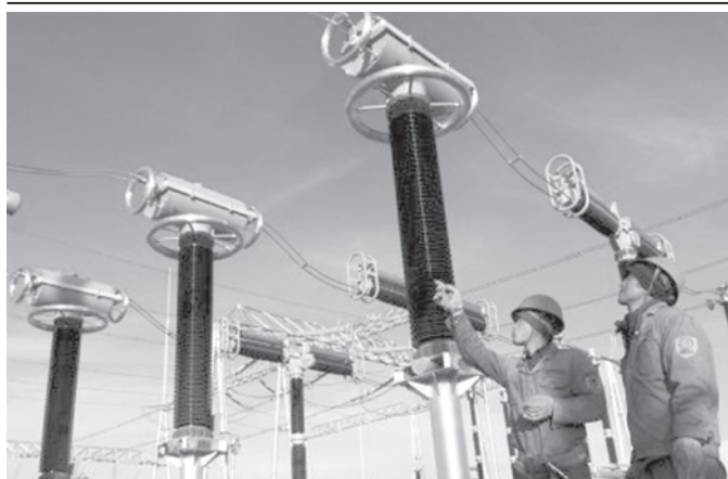
Two electricians conduct on spot technical inspection and debugging to the apparatus of the 330 kilovoltage booster substation, at the Jiuquan Dongfeng Electricity Generation Field, in Guazhou County of Jiuquan City, northwest China's Gansu Province, on 8 Dec, 2009.—XINHUA
