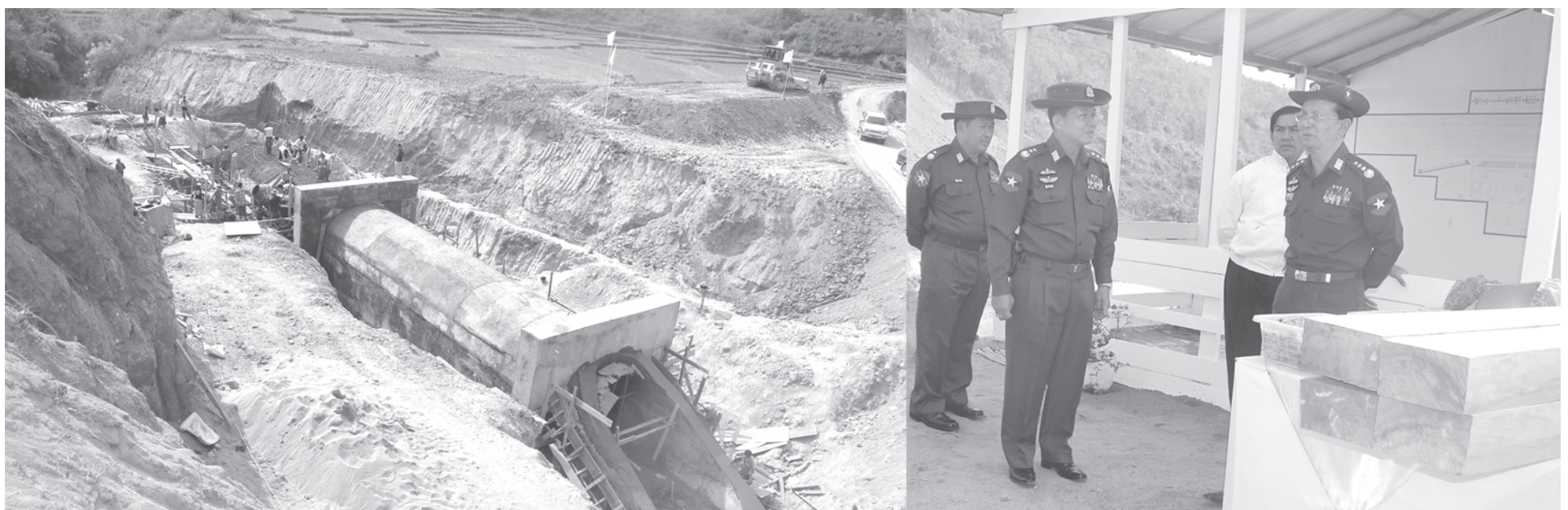
Prime Minister General Thein Sein inspects construction of a conduit for the railroad project on Hsinhnakaung Hill in Kengtung-Monghsat railroad section.—MNA
