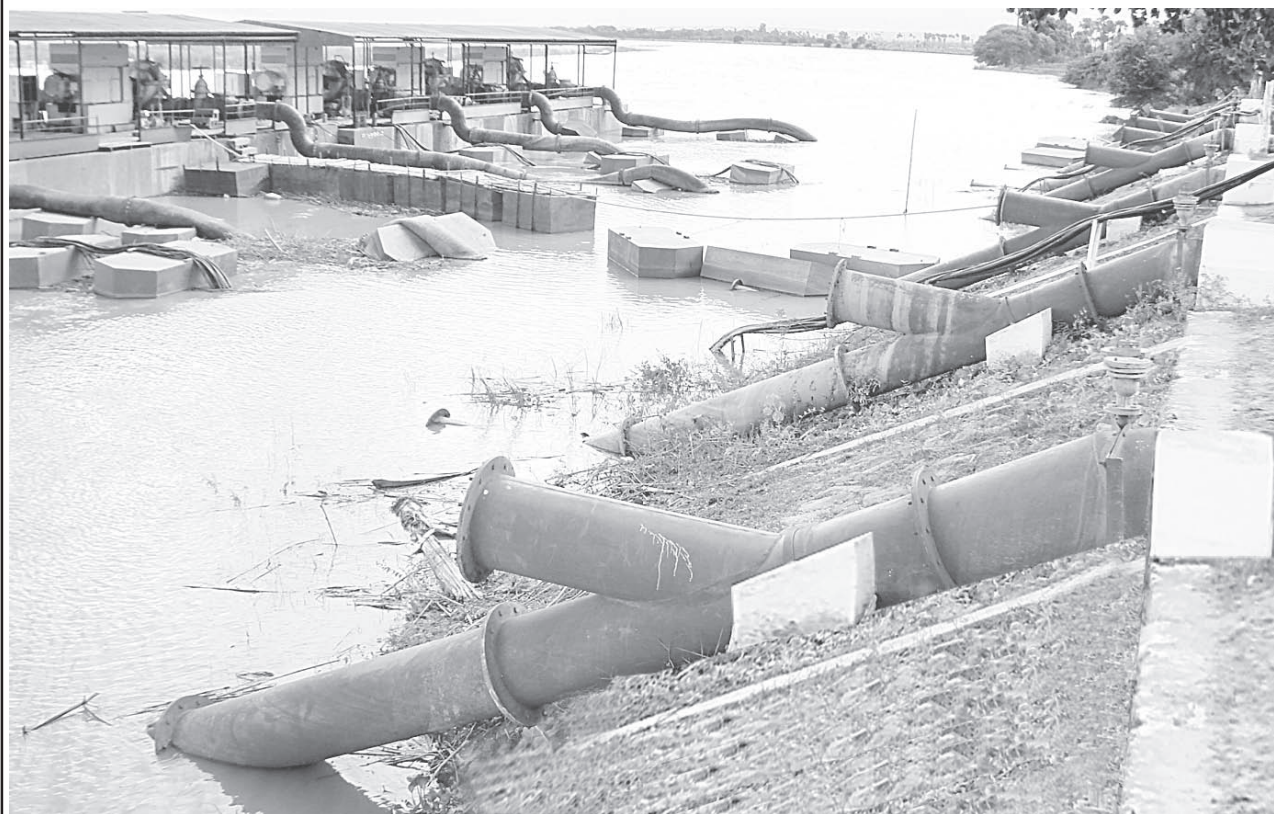
Tanyaung river water pumping station supplying irrigation water for Salin Township.
