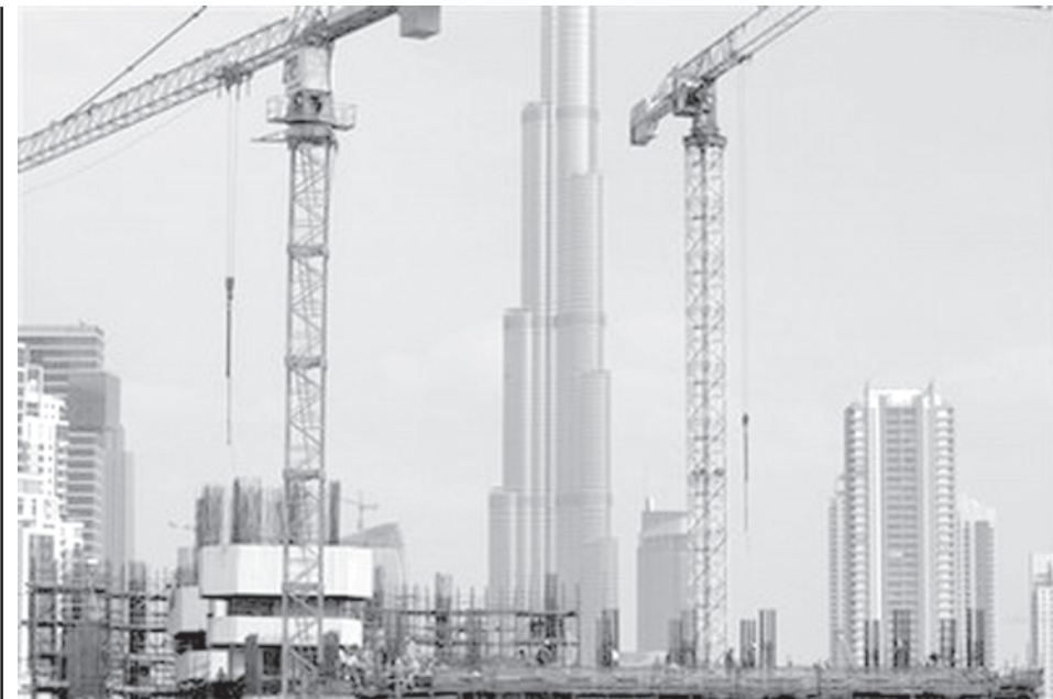
The Burj Dubai, the worlds tallest building under construction, is seen in the background as construction workers are seen at a site at the Business Bay district in Dubai, United Arab Emirates, on 30 Nov, 2009.
