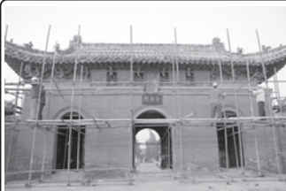
Workers build up scaffolding before starting restoration of the Taihao Mausoleum in Huaiyang County, central China's Henan Province, on 25 Nov, 2009. The emergency restoration of the Taihao Mausoleum was initiated recently and will be finished by the end of January 2010. The Taihao Mausoleum is believed to be the mausoleum for a legendary ancestor of the Chinese nation.
