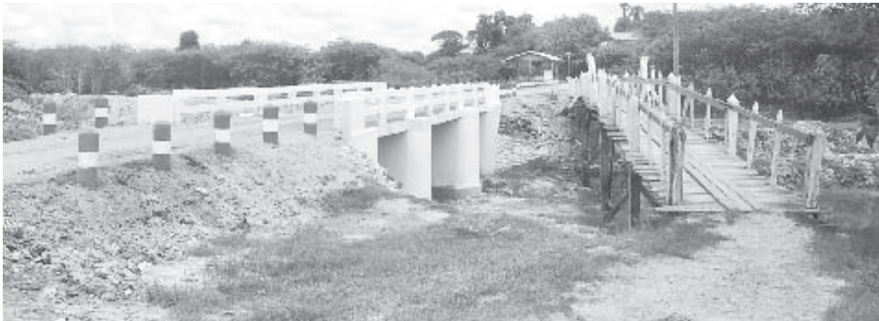
A concrete bridge is being built, shoulder to shoulder with the old wooden bridge in Kyudaw Village in Pyawbwe Township.
