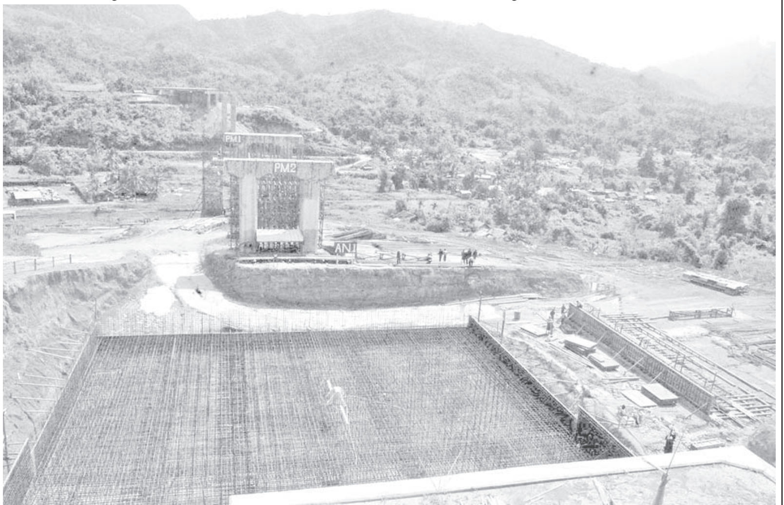
Photo shows construction of 1760 feet long suspension bridge on Nay Pyi Taw-Pinlaung Highway.
