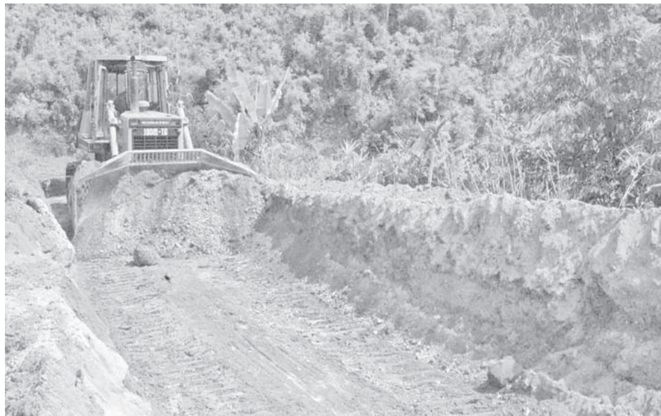
Construction of approach bridge with heavy machinery in progress at Leinli Bridge Project site.
