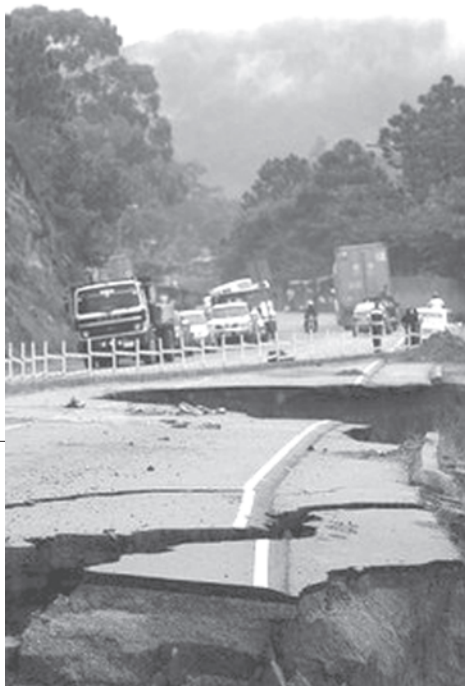
View of a damaged national road in the outskirts of Tegucigalpa, Honduras, in 2008. Central American nations will demand 105 billion dollars from industrialized countries for damages caused by global warming, the region's representatives said on Friday.—INTERNET
