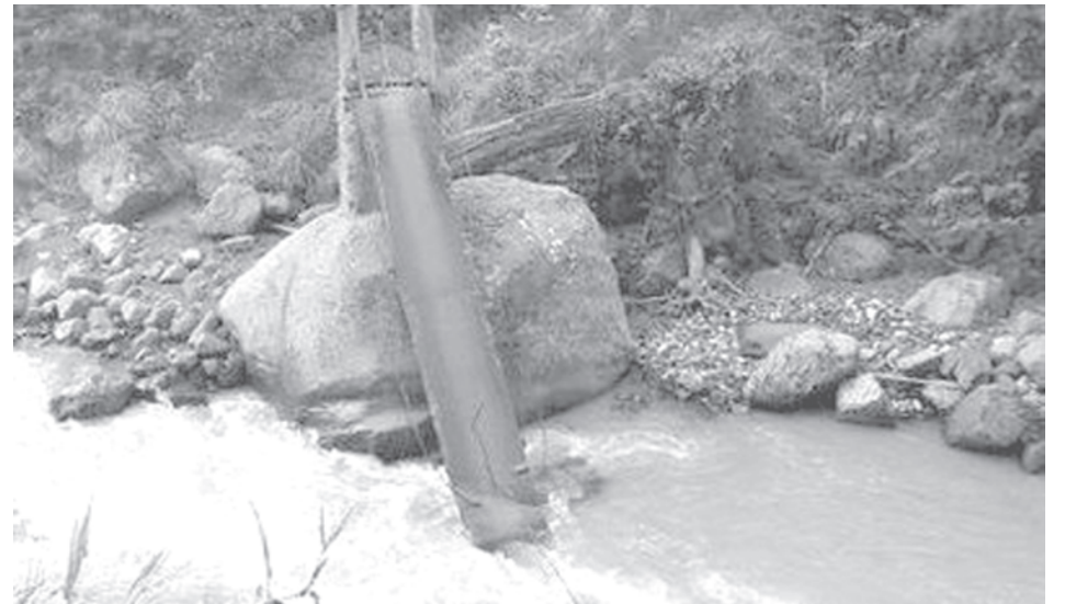
A bridge that crosses into Colombia's Norte de Santander department lies destroyed on 19 Nov, 2009.—INTERNET
