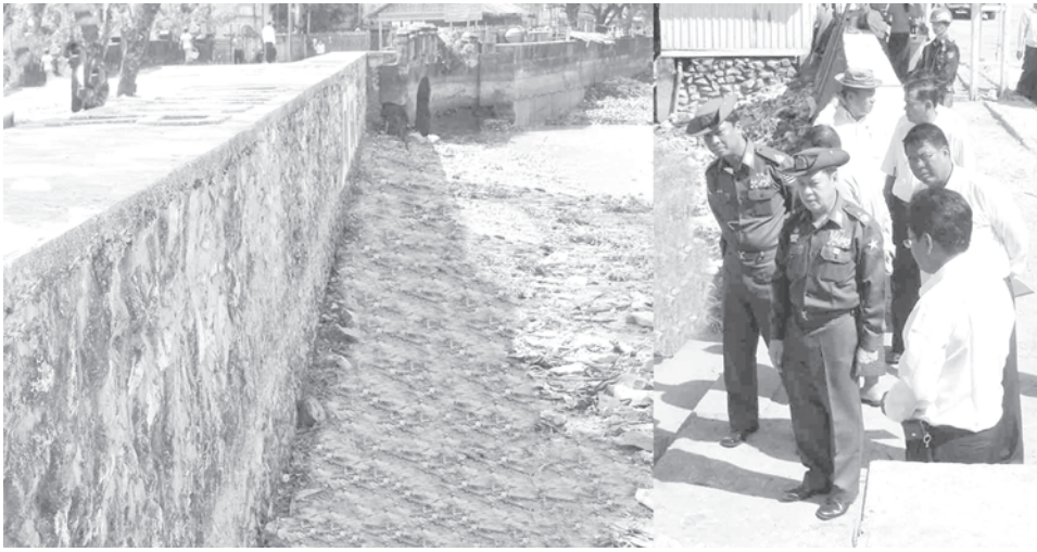
Commander Maj-Gen Kyaw Swe and Minister Maj-Gen Thein Swe inspect progress in construction of retaining walls on Strand Road in Ywe Bo Tat Ward of Patheingyi.—MNA
