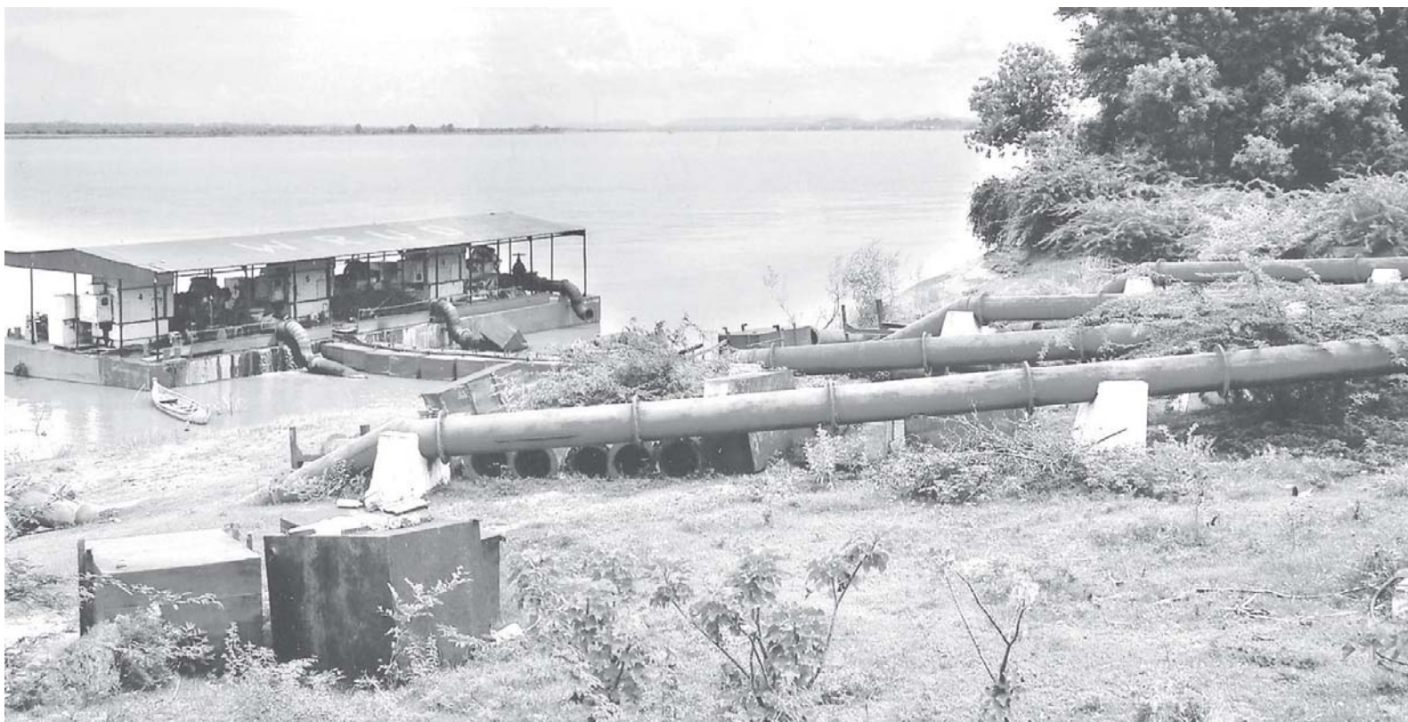
Umin Koepauk river water pumping station installed with water pipelines supplying water from Ayeyawady River to over 4700 acres of paddy and other crops in Chauk Township.
