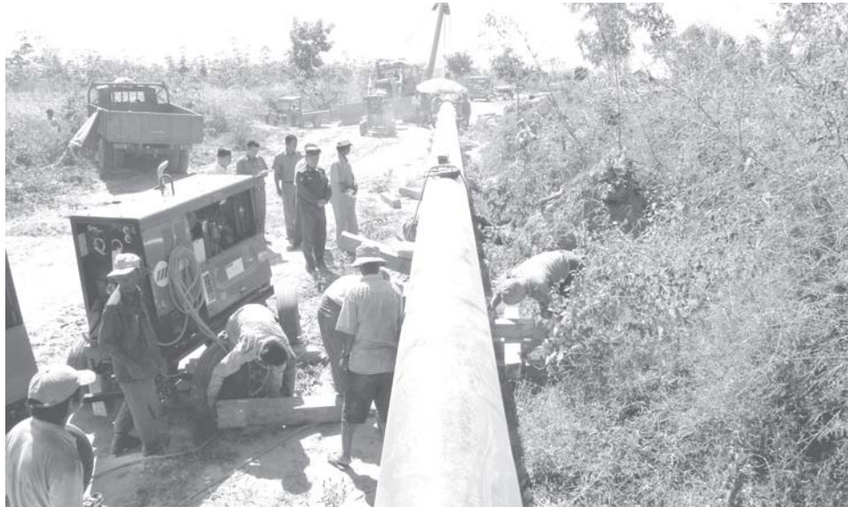
Minister for Energy Brig-Gen Lun Thi inspects laying of 24-inch diameter natural gas pipelines on Kungyangon-Twantay Tawgyidan section.—MNA
