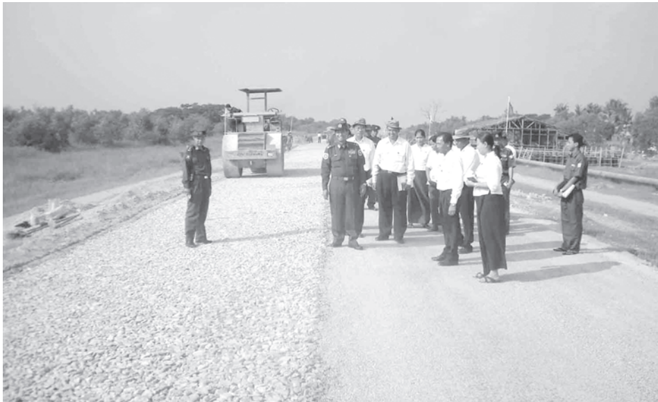
Minister for Construction Maj-Gen Khin Maung Myint inspects tarmacking of Dalla-Twantay Road.—CONSTRUCTION
