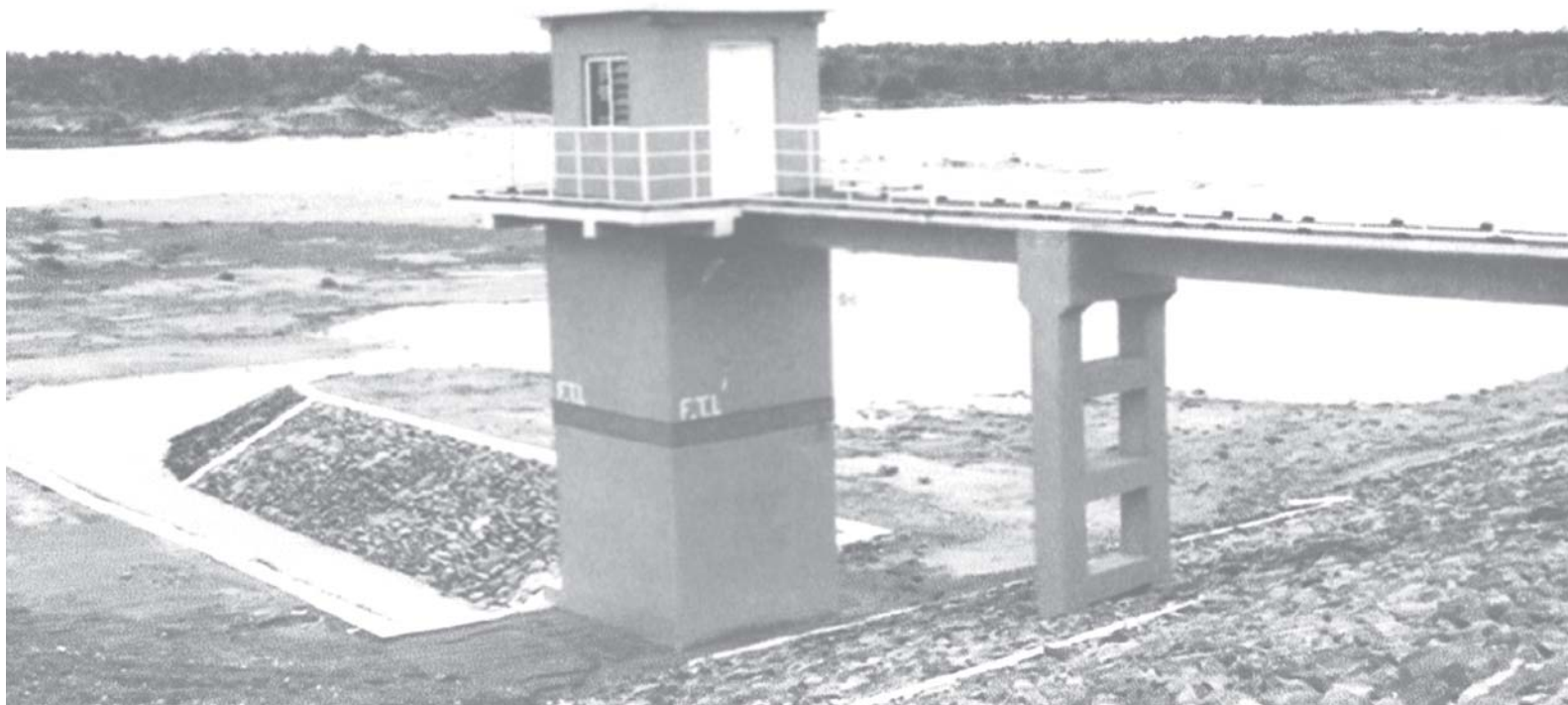
Water control tower of Ngachin Dam in Seikpyu Township of Pakokku District.
