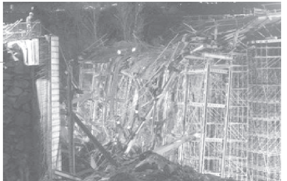
The construction site where a bridge collapsed in Massana near Andorre-la-Vieille. A bridge collapse in Andorra on Saturday killed at least three workers, left seven badly hurt and one missing, feared buried under the rubble, the government said.
