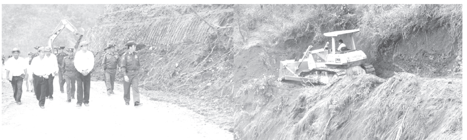
Lt-Gen Tha Aye inspects Gangaw-Haka road section at mile post No. 25.—MNA
