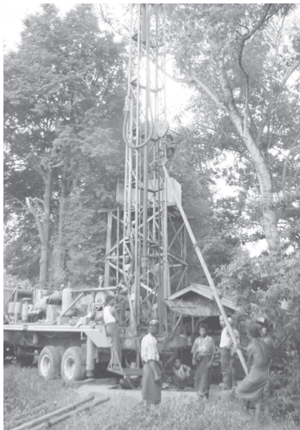
Sinking a tube-well in progress at Kyagan Village of Magway Township for supply of potable water to rural people.
