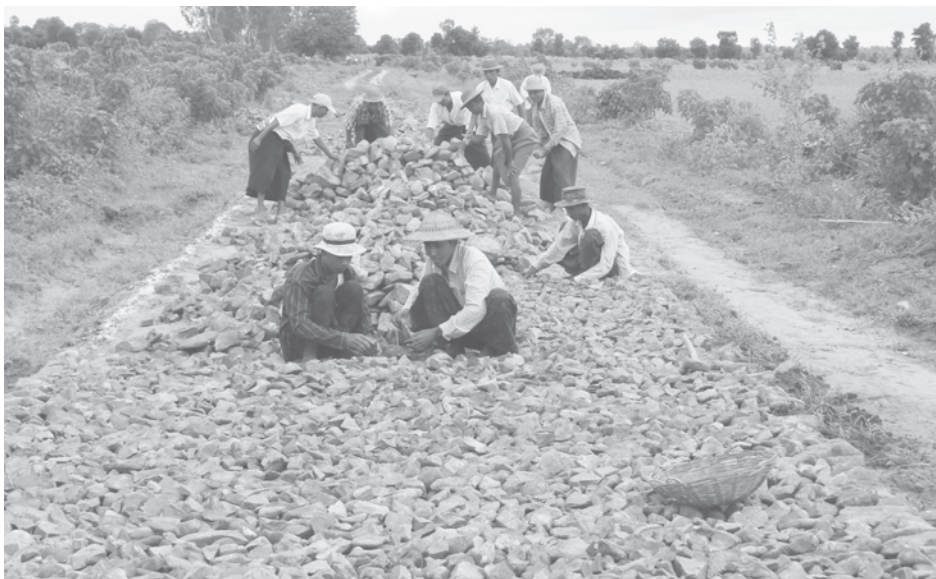
Workers seen at construction of gravel road to Hsugauksan Village in Magway Township.
