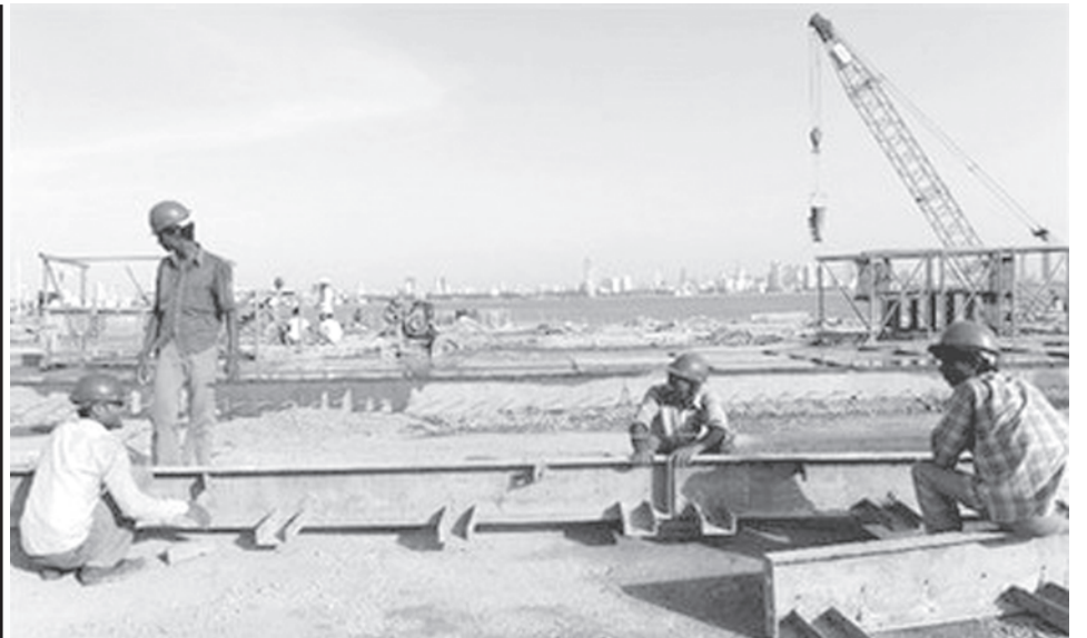
Workers are seen constructing a section of a new road in Mumbai. Thousands of foreign workers in India face a deadline on Saturday to be out of the country in a visa clampdown aimed at cracking down on tax-dodging expats and unskilled labour.—INTERNET
