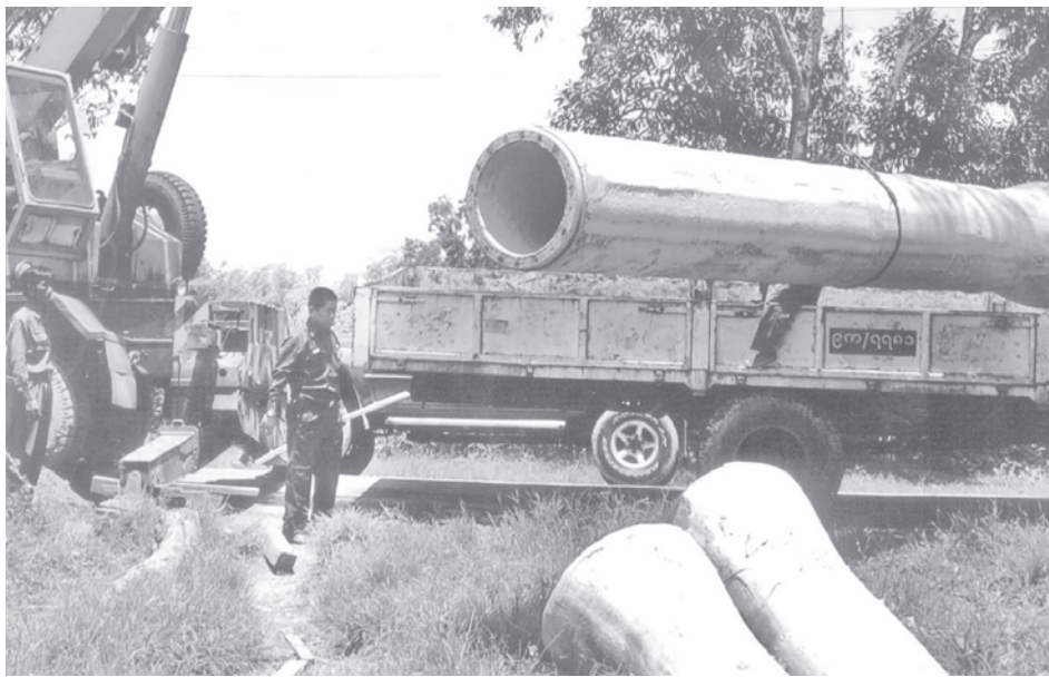
RC water pipelines being laid with the use of heavy machinery to supply water to Hlinethaya Township from Water Supply Project (Thebyu).
