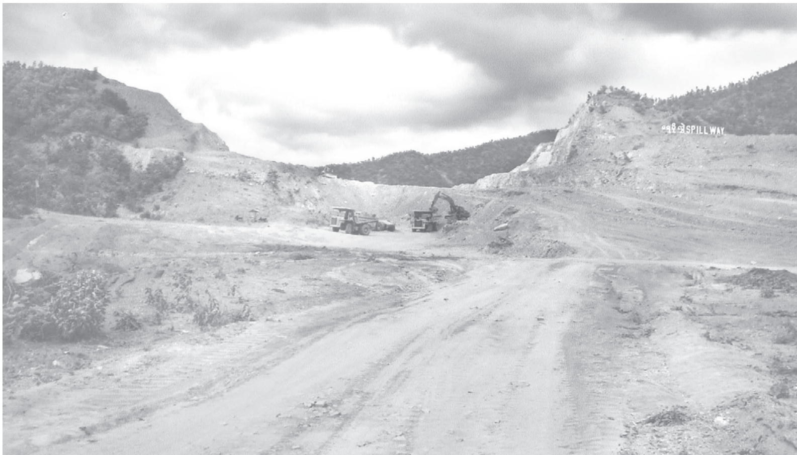
Some units of heavy machinery at work site to construct a spillway.
