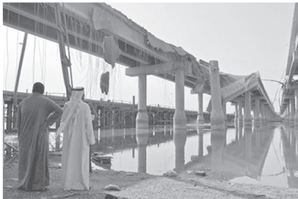
Iraqi men inspect a bridge destroyed in a truck bomb attack in Ramadi, 115 kilometers (70 miles) west of Baghdad, Iraq, on 17 Oct, 2009. A suicide bomber driving an explosives-laden truck destroyed a key bridge on Saturday on a highway used by the departing US military.—INTERNET
