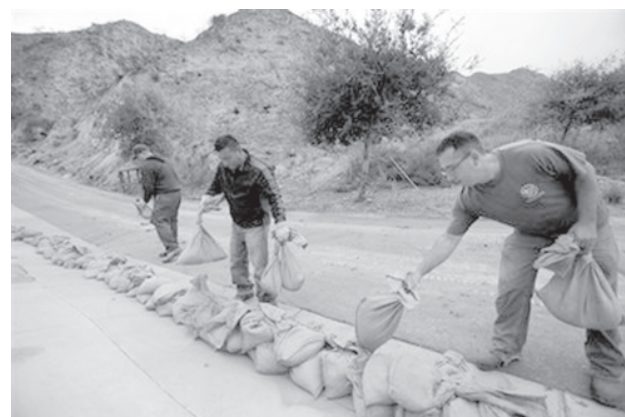
Workers with the City of Glendale Parks, Recreation & Community Services set sand bags at the Deukmejian Wilderness Park overlooking the foothill communities of La Crescenta and Tujunga, in Glendale, Calif on 12 Oct, 2009. Southern California communities near wildfire burn areas are preparing for the possibility of mudslides as a strong Pacific storm remains on course for the West Coast.— INTERNET
