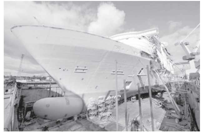
Allure of the seas, sistership of Royal Caribbean's Oasis of the Seas cruise ship is built at the STX Europe shipyard in Turku. The Turku shipyard specialises in large cruise ships, and the future of most employees there looks bleak. When Allure of the Seas, is delivered next autumn, most of STX's 2,300 employees in Turku will be temporarily laid off, the shipyard's director said.—INTERNET
