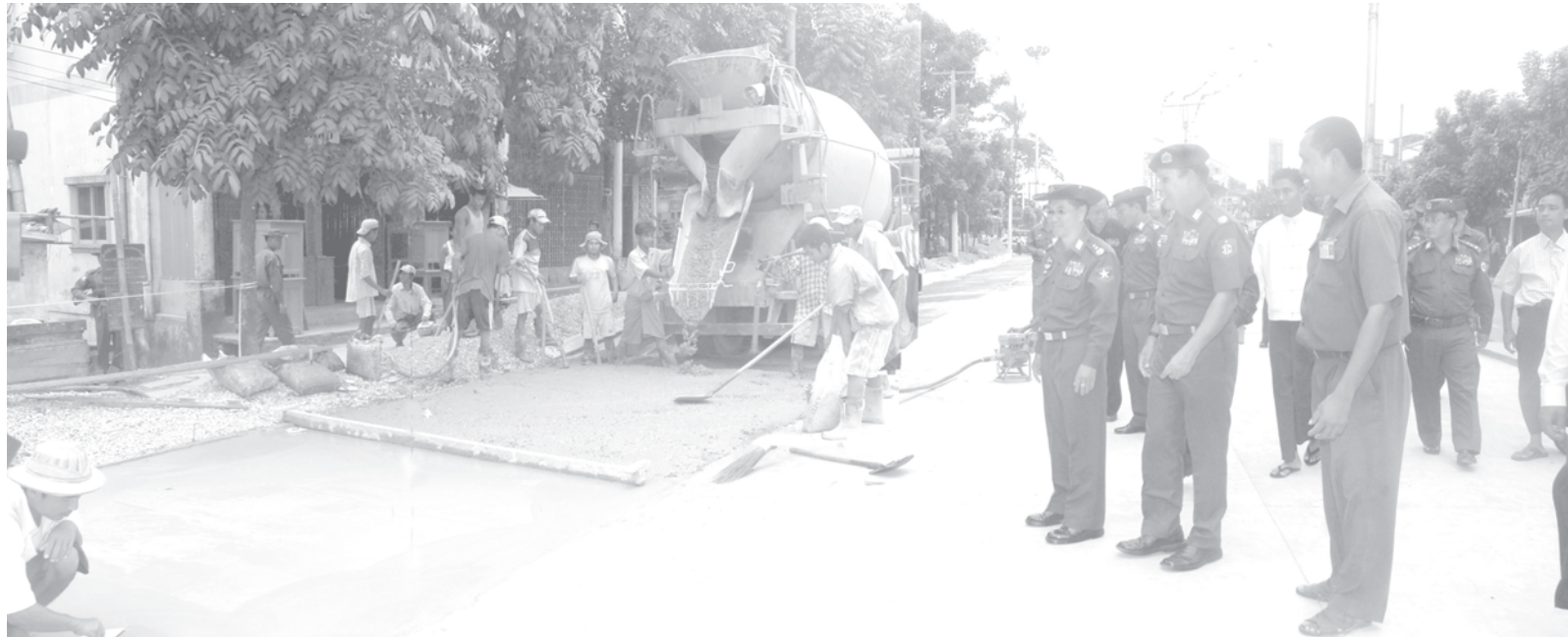
Lt-Gen Myint Swe inspects upgrading of Thameinbayan Road in Tamway Township. —MNA
