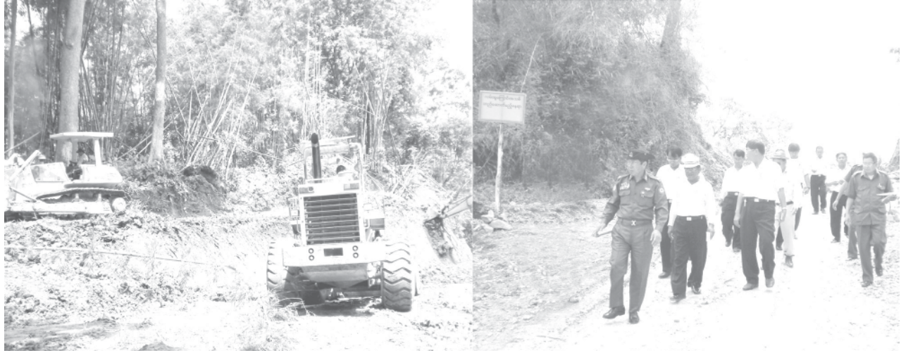
Deputy Minister Brig-Gen Myint Thein inspecting repairing of Pyay-Paukkaung-Toungoo (Ottwin-Paukhaung) road section.—CONSTRUCTION
