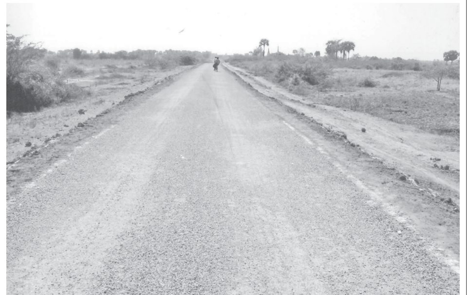
The road section between Mile Posts Nos 46/4 and 46/5 of No (1) Inter-District Road in Wundwin Township.
