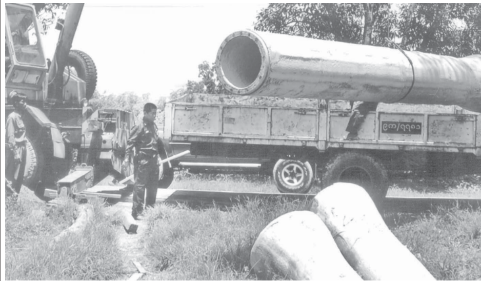
The laying of reinforced concrete pipe is in progress to supply portable water to Hlinethaya Township.
