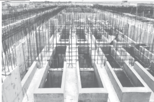
Collector tanks, filtering tanks and storing tanks are under construction in the second step of Yangon City Water Supply Project (Nga Moe Yeik).
