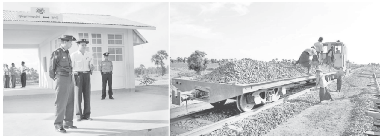
Minister Maj-Gen Aung Min inspecting construction of railway tracks and laying gravels at Begyi station.—MNA
