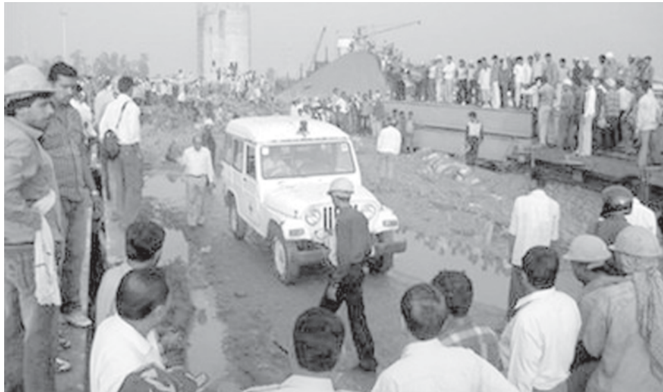
People gather at the site of a collapsed chimney in Korba on 23 Sept. The death toll from the collapse of a giant chimney in central India rose to 36 on Friday, with many more bodies set to be pulled from the debris, a local government official said.—INTERNET
