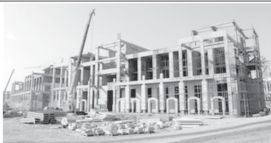
The construction site of the King Abdullah University of Science and Technology (KAUST) in Jeddah earlier this year. King Abdullah University is a research institution which has been launched this week. The aim of the University is to promote research and science achievement.—INTERNET
