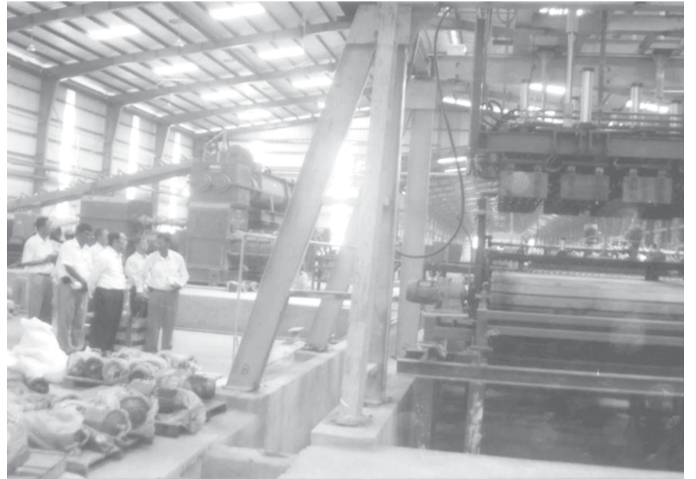
Minister for Industry-1 U Aung Thaug visits Nay Pyi Taw Brick Factory Project (Minkon).—INDUSTRY-1
