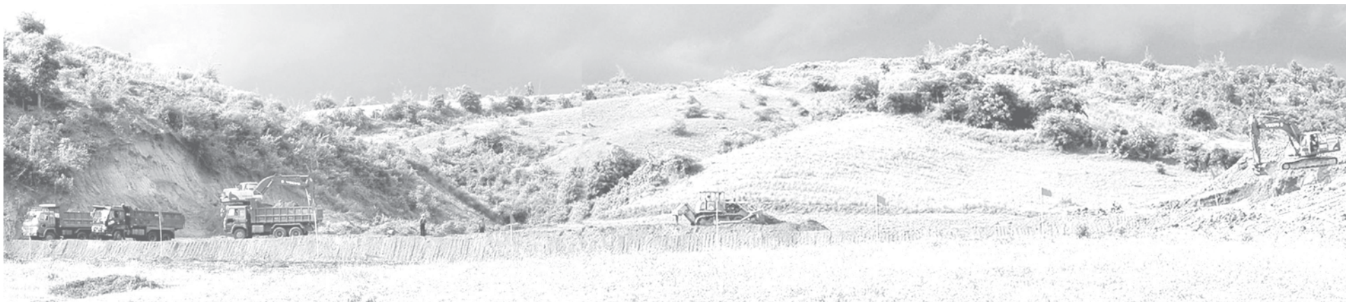
Earthworks in progress on Pyay-Paukhaung section of Pyay-Paukhaung-Toungoo-Nay Pyi Taw rail road.—MNA
