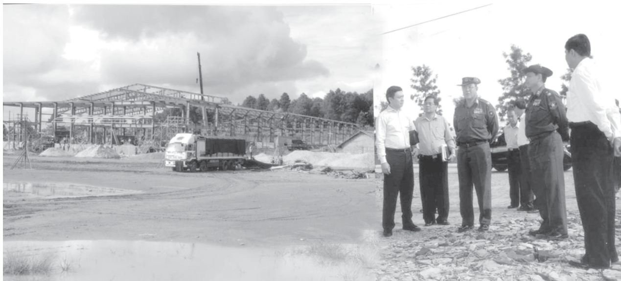
Minister for Communications, Posts and Telegraphs Brig-Gen Thein Zaw views progress in construction of Soft Base Factory in Yatanarpon Myothit, PyinOoLwin Township.—MNA
