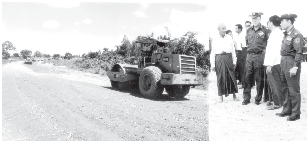
Minister for Communications, Posts and Telegraphs Brig-Gen Thein Zaw and Minister for Livestock and Fisheries Brig-Gen Maung Maung Thein inspect construction of Myitkyina-Tanai road section.—CPT
