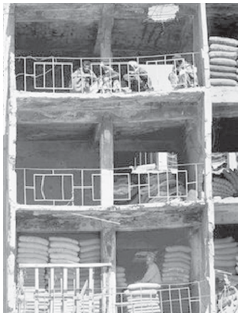
Traders stock their goods in the shell of a rocketed building in Kabul. A rocket fired on a house in Kabul in the early hours of Monday morning killed three members of one family and injured two others, officials said.—INTERNET
