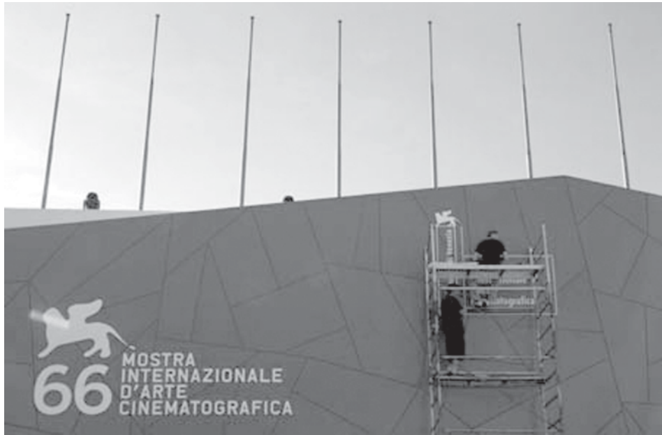
Workers give the final touches to the front entrance of the Cinema Palace in Venice on 31 Aug, 2009. The 66th Venice Film Festival will take place from 2 September to 12 September, 2009.—XINHUA
