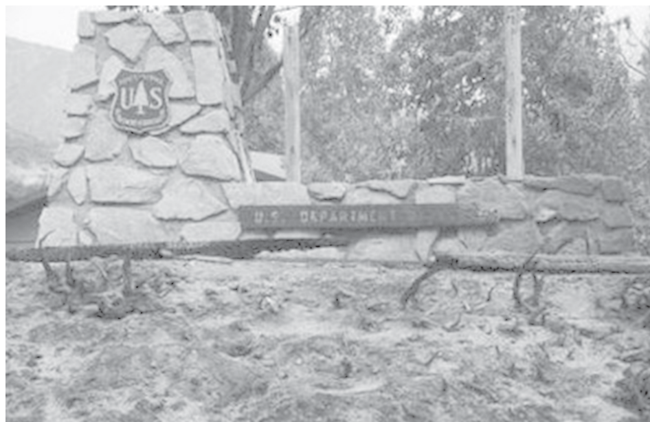
Angeles National Forest Monte Cristal Ranger Station is destroyed during day seven of the Station Fire in California On 1 September, 2009. Firefighters took advantage of a turn in the weather on Tuesday to gain ground against the enormous wildfire burning for a week above Los Angeles, saying they now hoped to drive the flames away from historic Mount Wilson, a key telecommunications site.—INTERNET
