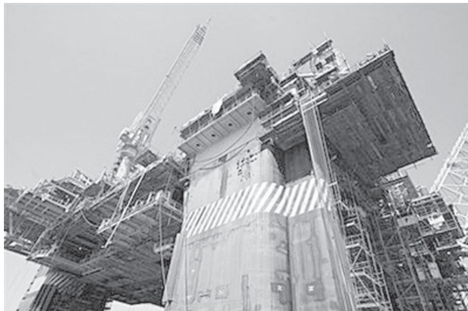
Partial view of the Petrobras P-51 semi-submersible off-shore oil platform under construction at the Brasfelf shipyard in Angra dos Reis, 180 km south of Rio de Janeiro, Brazil, in 2008. Brazil is to boost state control of vast, recently discovered offshore oil fields by giving its oil company Petrobras a minimum 30 percent stake in areas open to foreign company exploitation.—INTERNET
