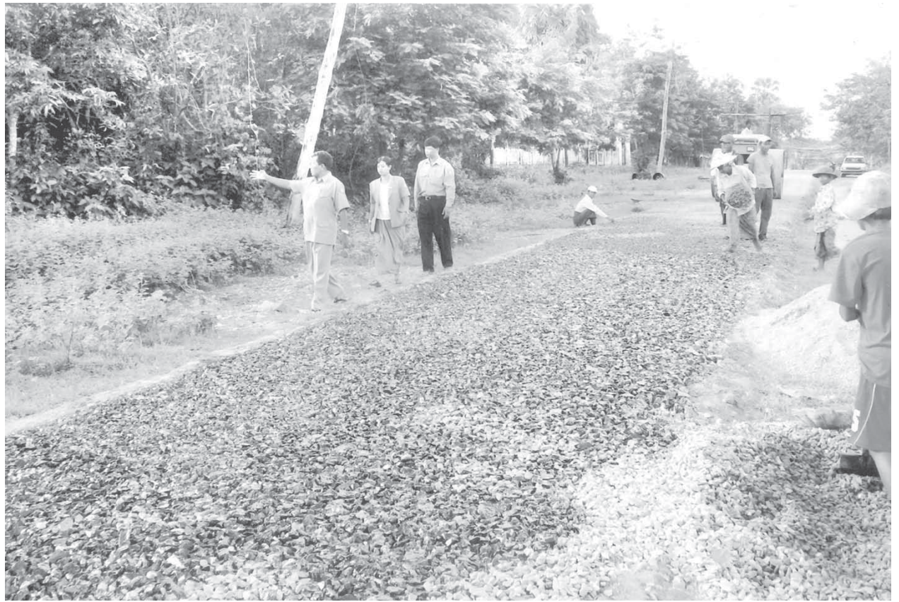
Executive Officer U Tun Myaing of Bago Township Development Affairs Committee and personnel supervising upgrading of Bayintnaung Road into tarred one.
