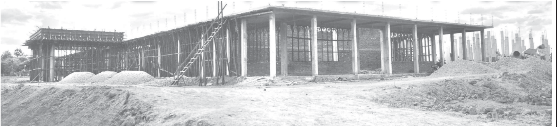
Construction of the Out-patient Ward of Kanbalu Township 100-bed Hospital in progress.
