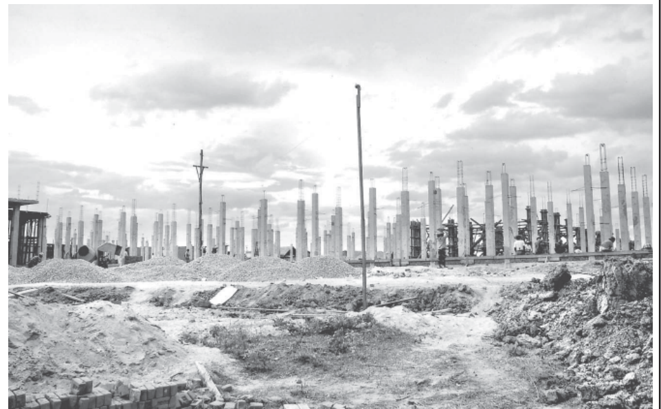
The construction site of a new building of Kanbalu Township 100-bed Hospital.
