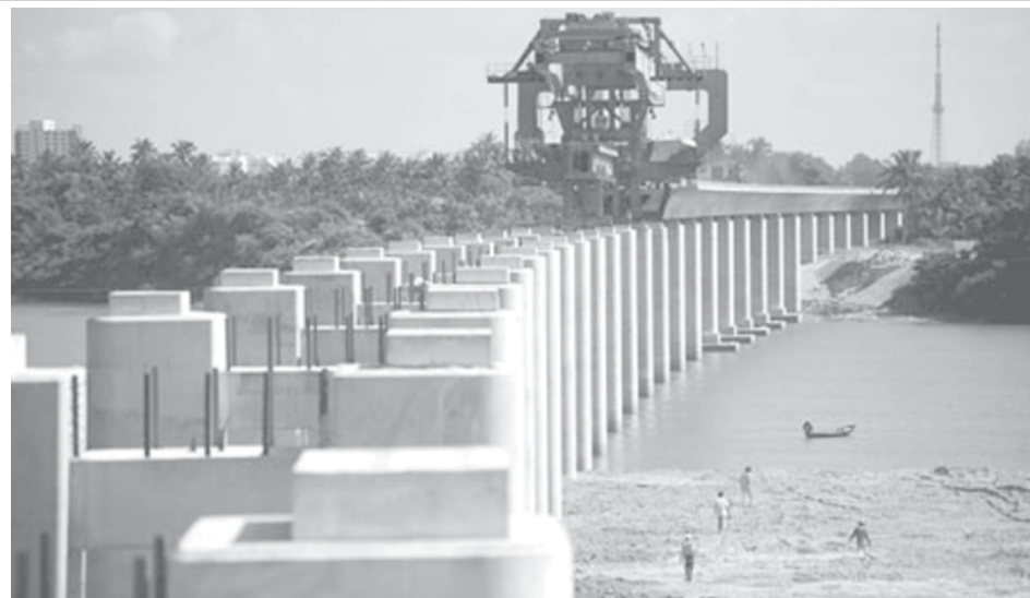
Box girders of the East Loop Railway are being installed at the work site of Wanquanhe Bridge in Qionghai City of south China's Hainan Province, on 22 Aug, 2009. A total of 122 box girders needed to be installed on the 3974-meter-long Wanquanhe Bridge, a section of the East Loop Railway of Hainan Province, which was started in Sept. of 2007 and planned to be completed in late 2010.—XINHUA
