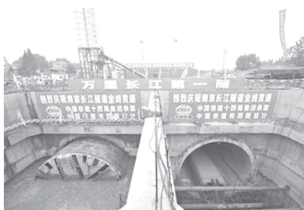
The finishing ceremony of a 6,042-meter six-lane traffic tunnel under the Yangtze River is held in Nanjing, capital of east China's Jiangsu Province, on 22 Aug, 2009.—INTERNET
