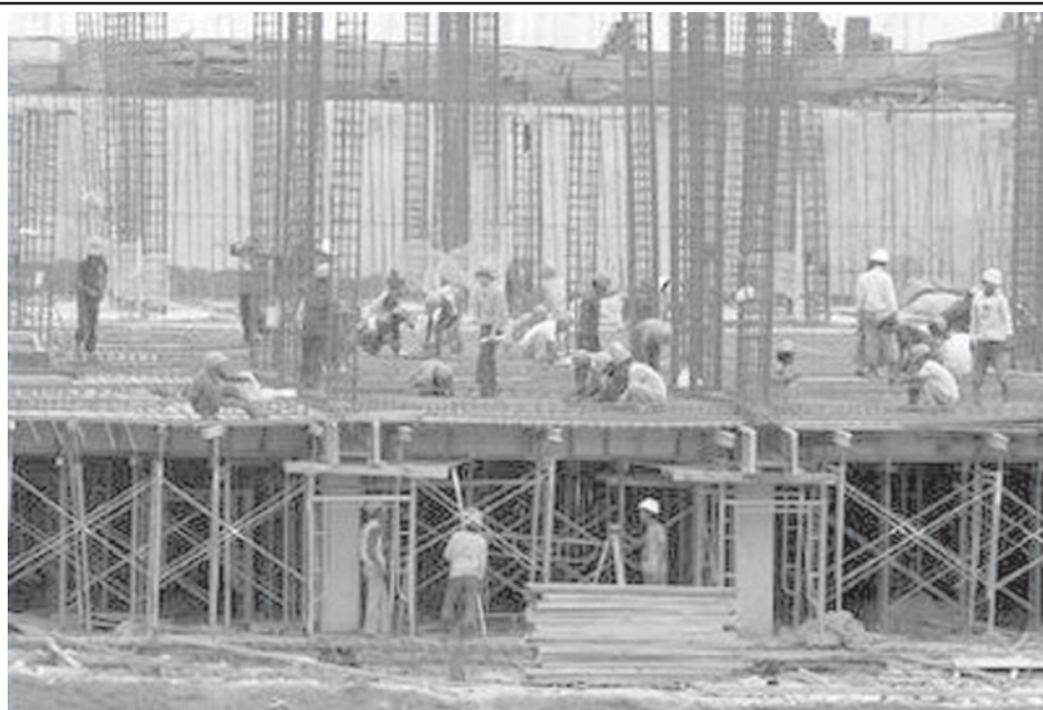
Labourers work on an apartment building construction site in Jakarta on early August, 2009.—INTERNET
