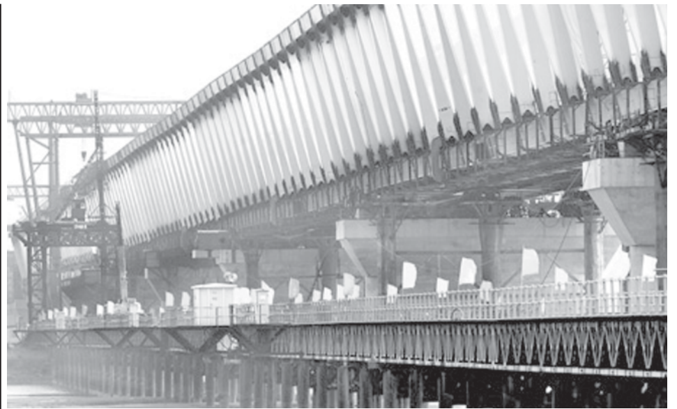
Photo taken on 13 Aug, 2009 shows the dual rail-road Yellow River bridge under construction in Zhengzhou, capital of central China's Henan Province. The construction of the dual rail-road Yellow River bridge will be completed in May 2010. —XINHUA
