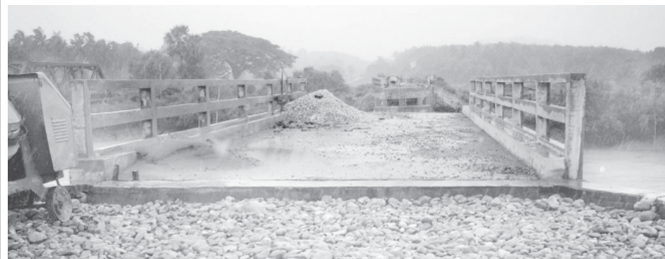
Construction site of Kayokepi bridge linking Kayokepi Model Village and Panga Village.
