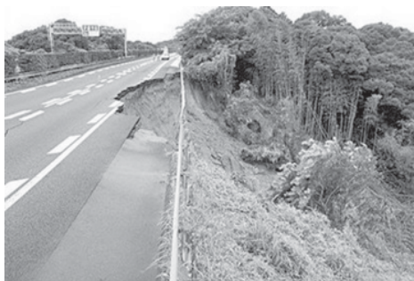
A collapsed section of the Tomei Expressway in Makinohara, west of Tokyo, after a strong earthquake left one person dead and 120 injured on 11 August. Another earthquake hit central Japan, including Tokyo, on Thursday, the Japan Meteorological Agency said.—INTERNET
