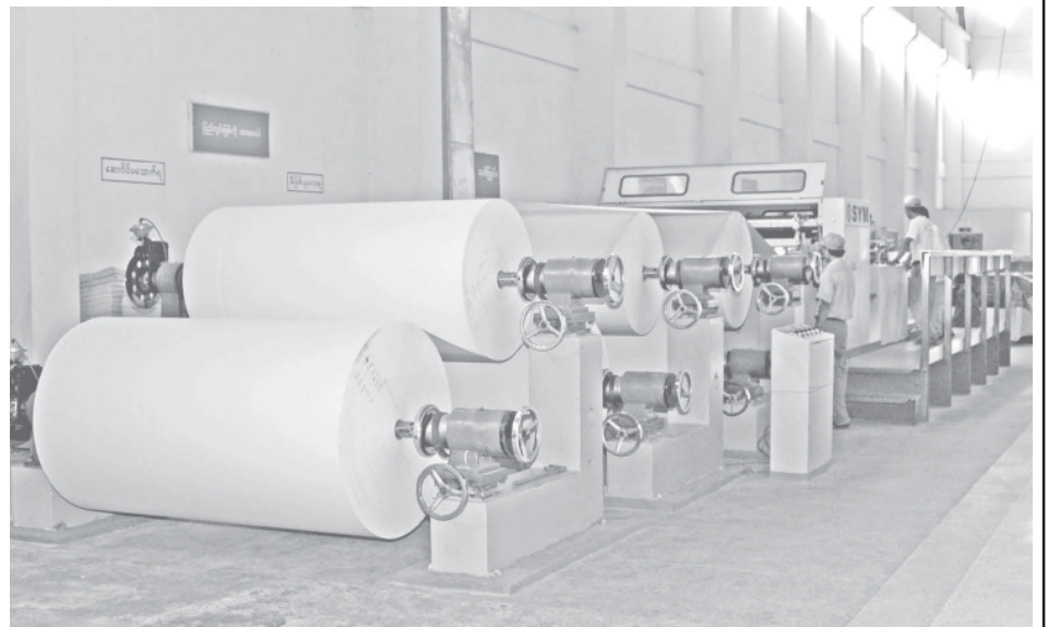
Production process of paper at the 50-ton Paper Mill (Thabaung).
