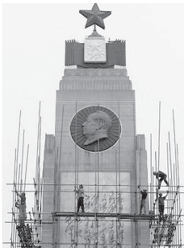
Workers install scaffolding as they carry out renovation work at a monument with an image of China's late Chairman Mao Zedong in Wuhan, Hubei Province on 11 August, 2009.
