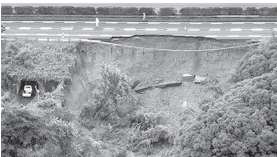
The shoulder of an express way is caved in after a magnitude 6.6 earthquake hit the area in Makinohara, west of Tokyo on 11 Aug, 2009. The powerful earthquake with a preliminary magnitude of 6.6 hit Tokyo and nearby areas shortly after dawn on Tuesday, halting trains and forcing two nuclear reactors to be shut down for safety checks.—INTERNET
