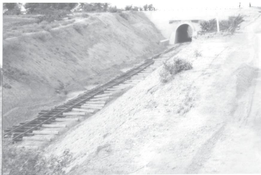
Minister Maj-Gen Aung Min views construction of roads, bridges and stations on Pwintbyu-Pakokku railroad section.—MNA
