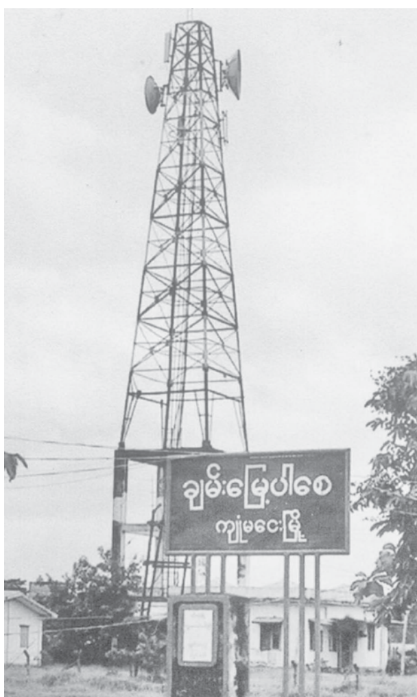
The microwave station of Kyonmange is for comfort and convenience of local people in communication.
