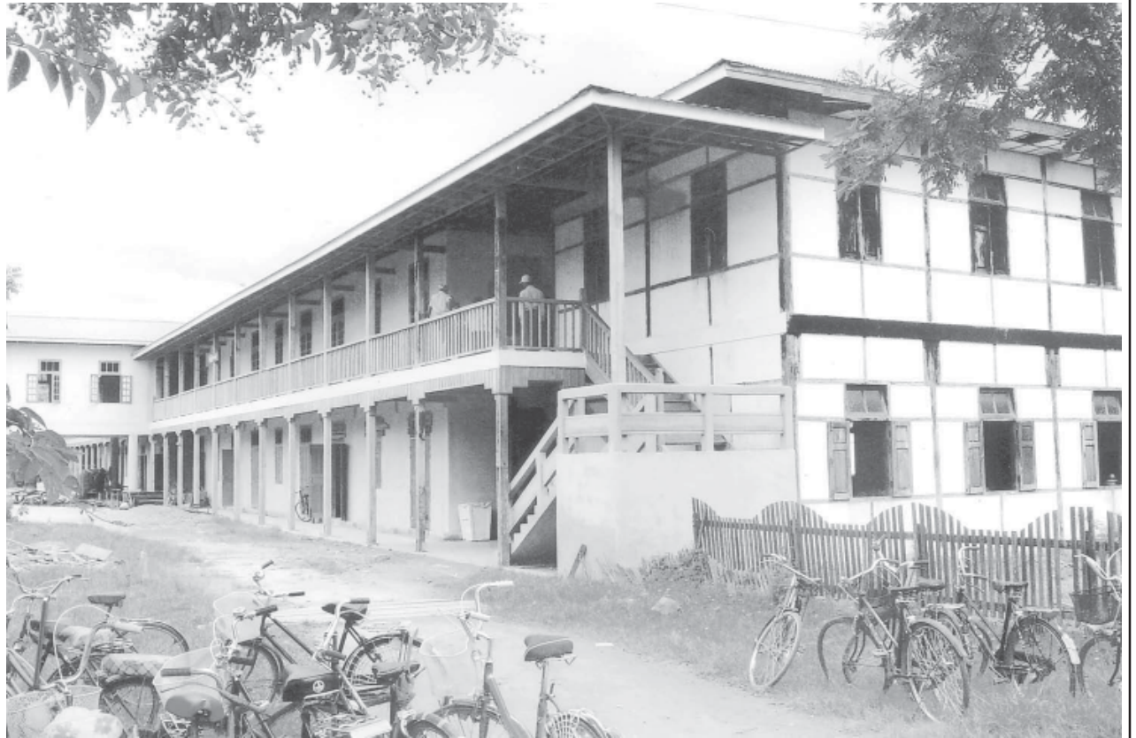
A new two-storey building under construction in Hopang Basic Education High School.
