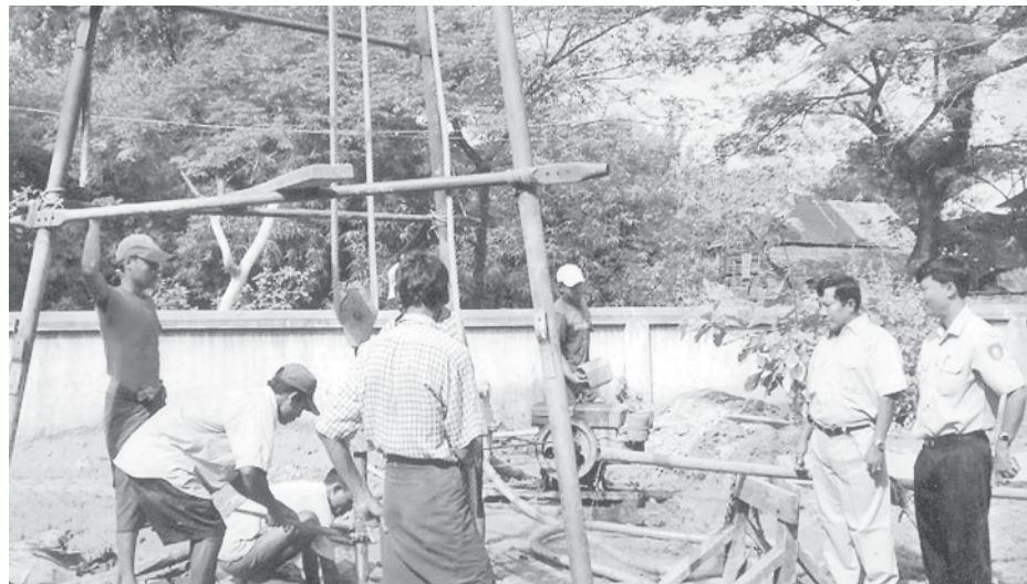
Township DAC sinking a tube well for Taunggyikwe Village in Bago Township.
