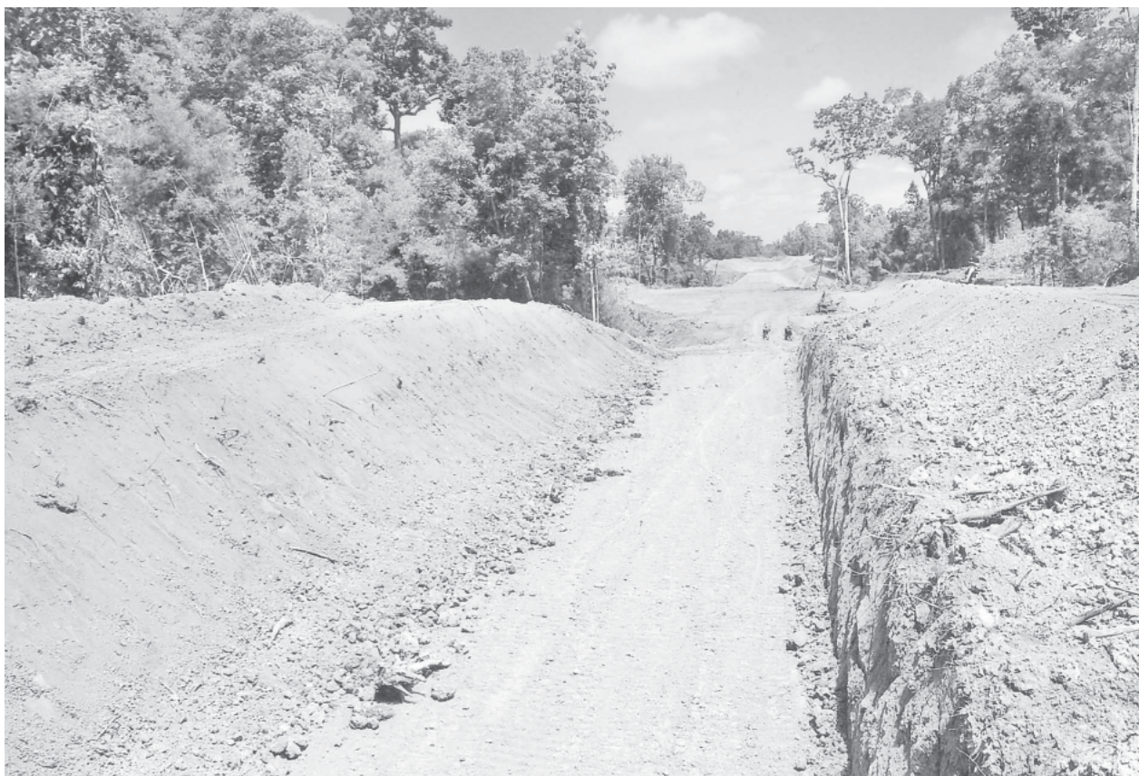
The axis of Bhamo-Katha Railroad near Kyaukkyi Village, Shwegu Township, Kachin State.
