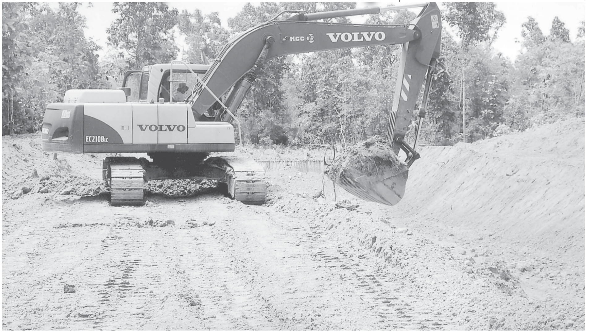
A unit of heavy machinery building the axis of Bhamo-Katha Railroad near Kyaukkyi Village, Shwegu Township, Kachin State.
